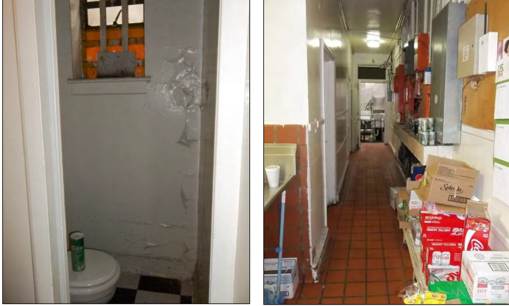
Photo 16: At Left, View of Staff Restroom, and at Right, View of Hallway Leading from Kitchen to Storage Spaces and Terminating at West-Side Kitchen Addition.
